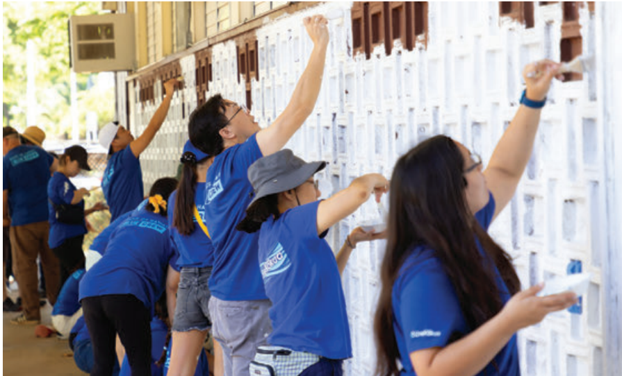
Our Blue Crew worked together to clean the campus of Princess Ruth Ke'elikōlani Middle School, including priming and painting walls, power washing sidewalks, gardening and picking up trash.
